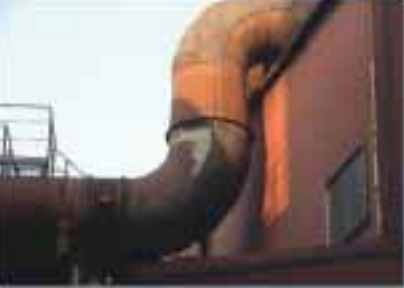
Coke Plant Pipe Elbow
