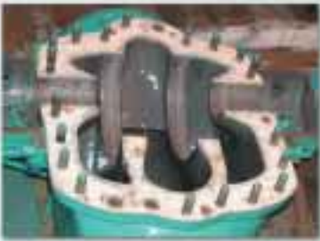
Reclaiming totally eroded surface
