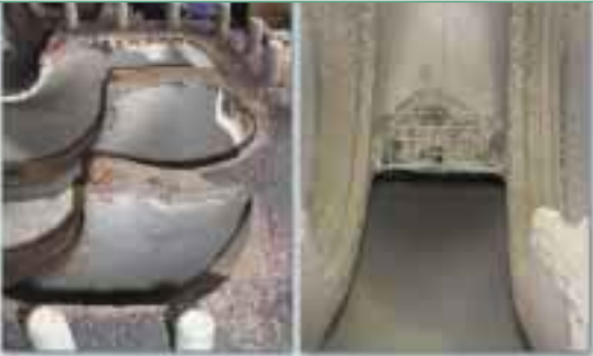
Pitting and erosion was clearly evident
